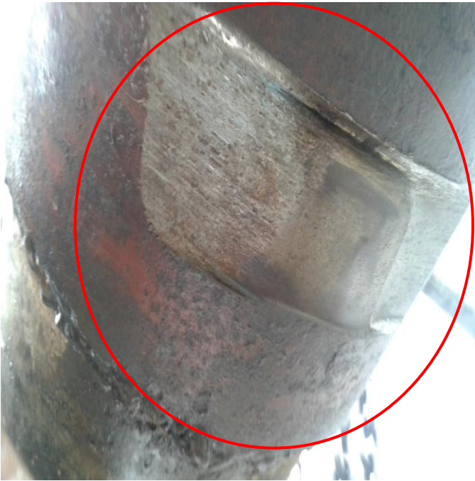
Fig A: The Incident Facility/Leak Point
